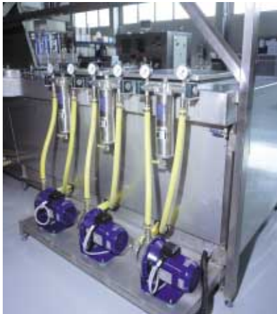
Closed loop particle filtration with 10' cartridge filters.
